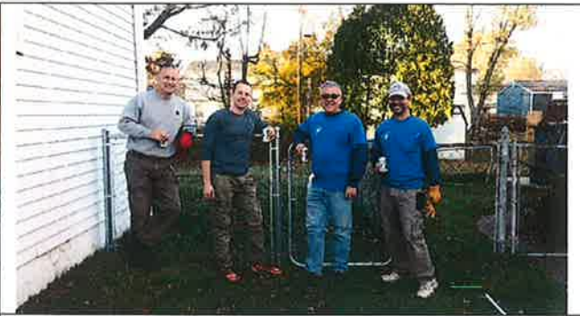
Tom Foos, Dale Galion, Bruce Jackson, and Rocky Lomano relax after installing fencing for a Parishioner in Need
