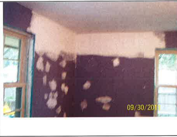
Walls were restored in two bedrooms and insulation was placed in all exterior walls of the house
