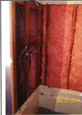
The master bathroom was gutted and new pipes and drains were installed. The new electrical load center is on the left side of photo. The new shower base and exterior wall insulation can also be seen
